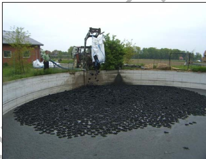
Figure 4.73: Load operation of floating bricks into a slurry tank (Hexa-Cover)
