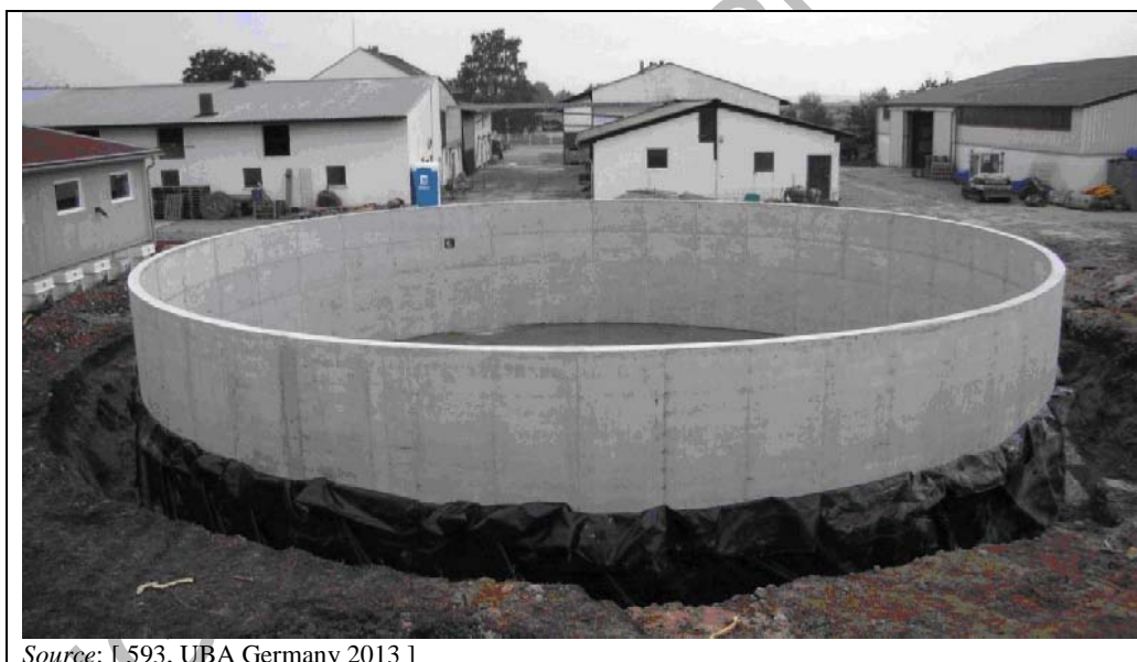
Figure 4.74: Below-ground slurry tank with liquid-tight geomembrane
