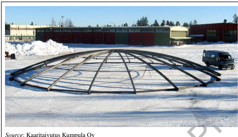
Figure 4.72: Dome-shaped steel structure for a flexible tent before its placement over the slurry store.
